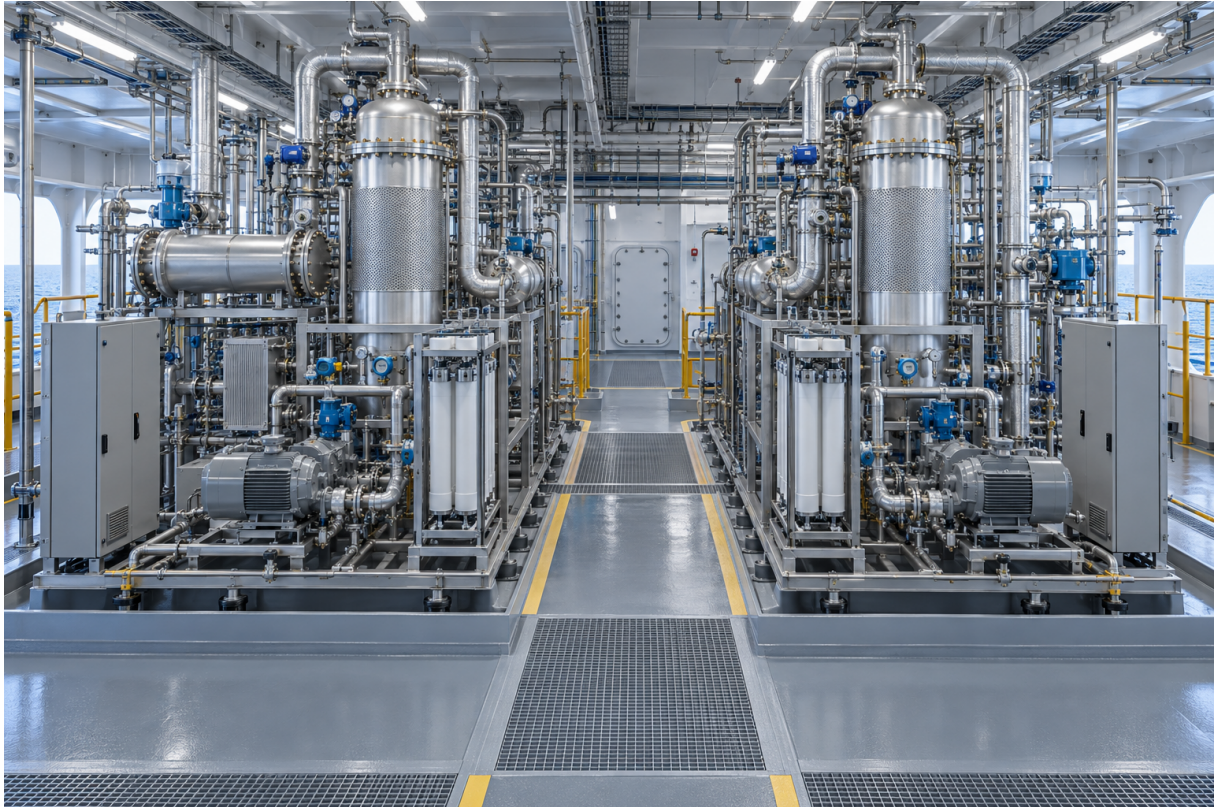
Figure 4.1: Conceptual equipment-room view of the redundant ammonia-cracking and hydrogen-purification trains.
